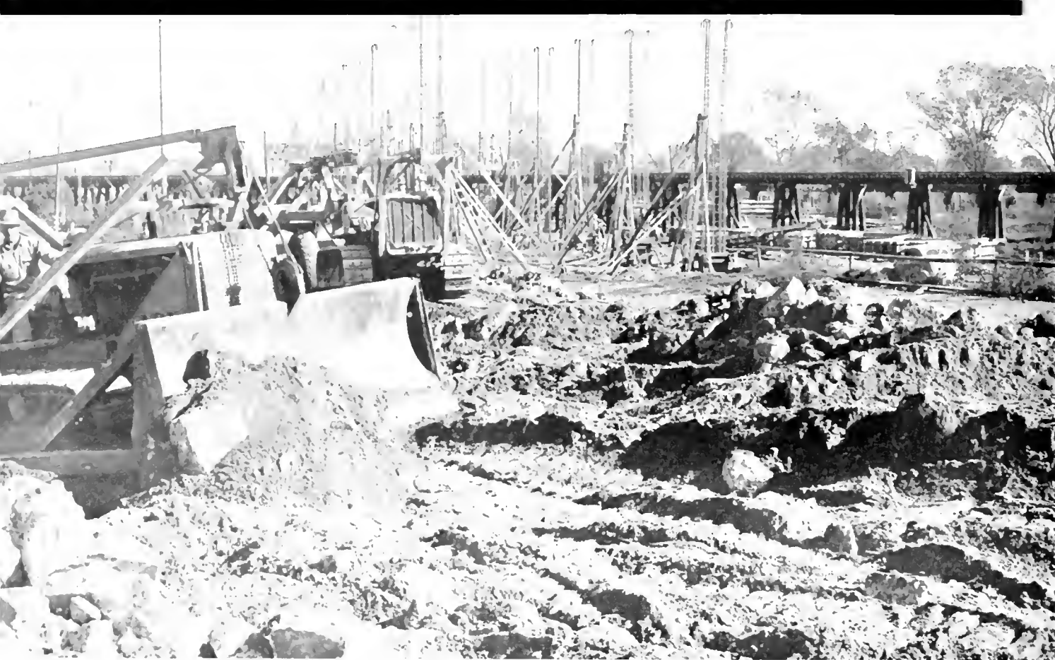
Equipment tearing up old pavement and grading for south approach to new North Sacramento Viaduct structure.
